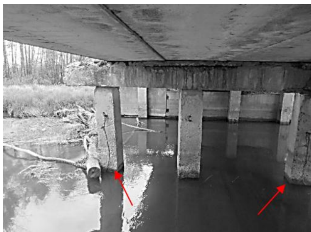
Fig. 1. Corrosion damage to reinforced concrete bridge structures in the Ivanovo region
