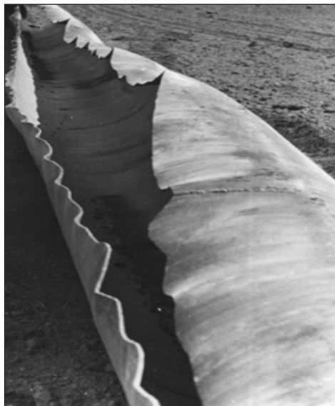
Fig. 1. Long crack on pipeline
